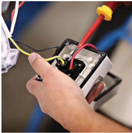
Data cabling and power outlets Eyecare Plus Mitcham
