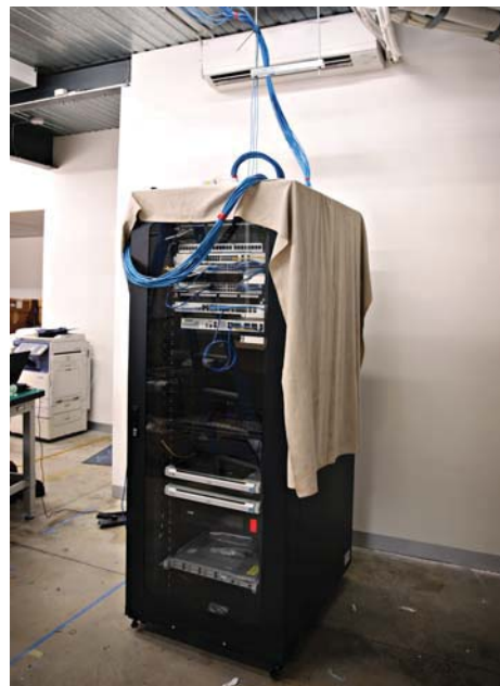
Data cabinet and Cat6 data cabling throughout the building installed WEBEX Board. ArchiTech Network & Communications Solutions
