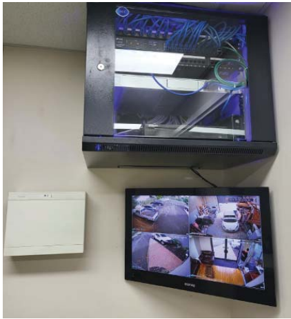
Monitor installations with client scheduling interface Alkira (Not for Profit)
